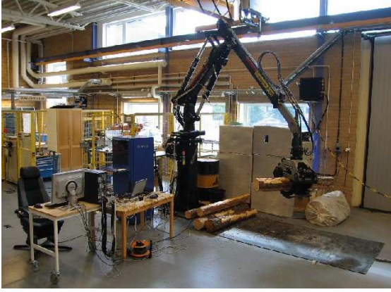
Fig. 2. Crane installed at the Department of Applied Physics and Electronics, Umeå University.
