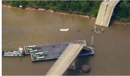
Figure 1.2 Barge-Impacted I-40 Bridge, Oklahoma, May 26, 2002
