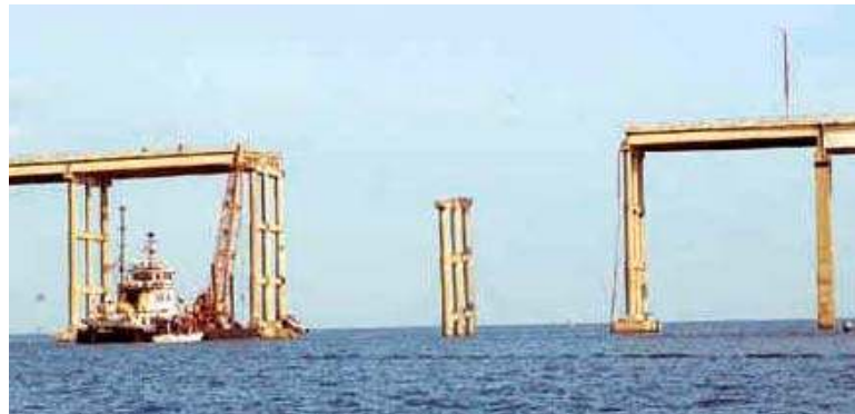
Figure 1.1 Four loaded barges crashed into the Queen Isabella Causeway, Texas, September 15, 2001, destroying a 73.2m (240 ft) section of the bridge
