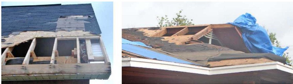
Fig. 1. Roof sheathing failures of houses in Hurricane Katrina (reprinted from van de Lindt et al. 2007)
