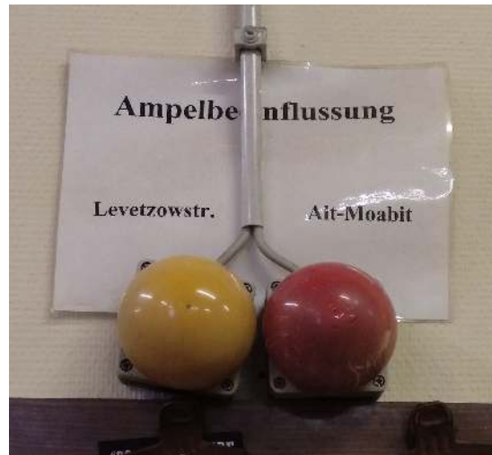
Figure 2: Example of a manual traffic management solution for emergency vehicles in a fire brigade in Berlin
