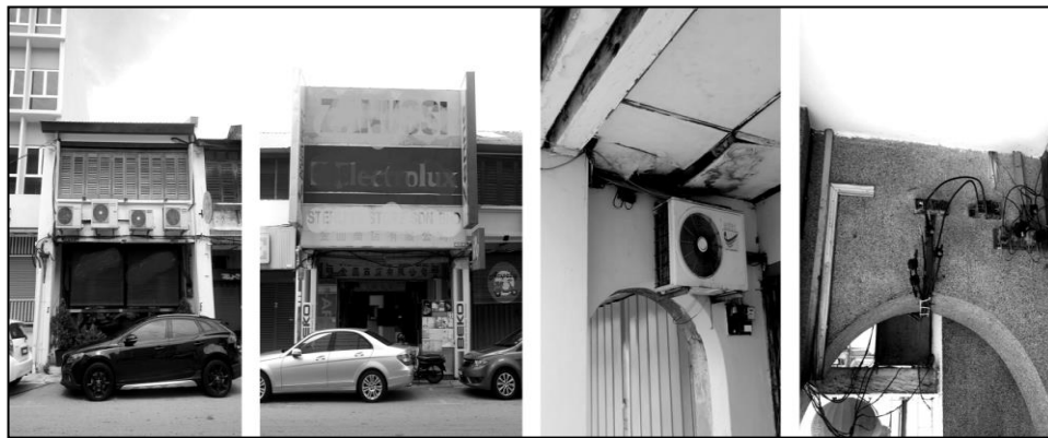
Figure 05. Samples of problems cause by modern building services
