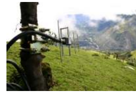
(c) Yagi antenna oriented towards observatory.
