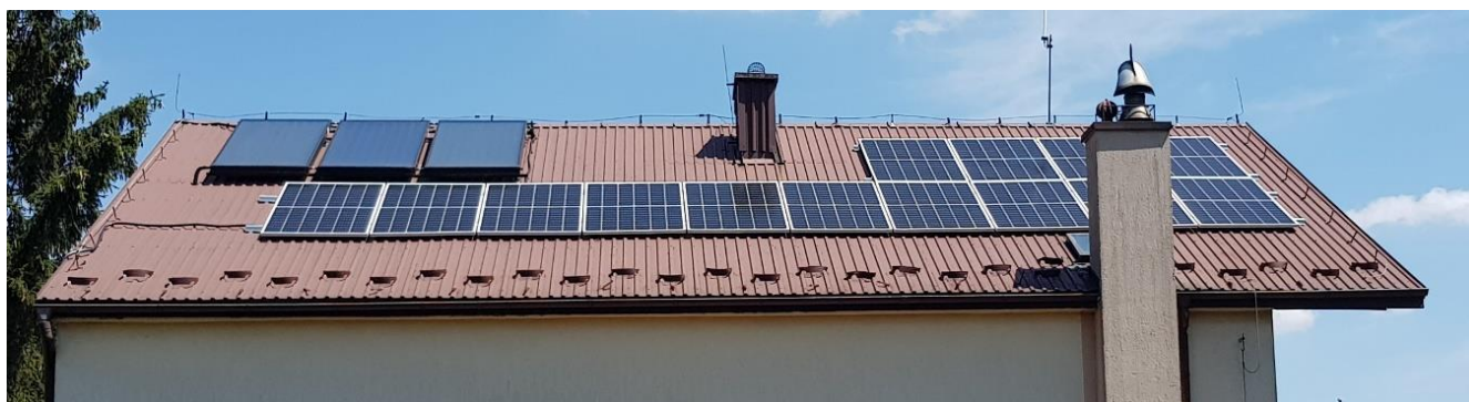
Figure 6. Panels on the roof of a single-family building in Leki.
