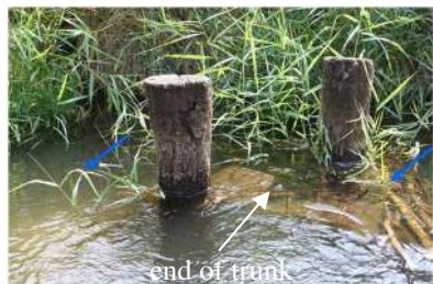
Fig. 6. Scour and flow at the wooden groyne toe.
