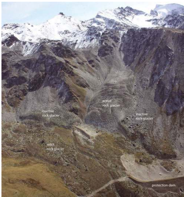
Fig. 8. Avalanche deflection and protection dams constructed in contact with relict, inactive and active viscous flow features of mountain permafrost, i.e. striking landforms resulting from cumulative straining by long-term creep of ice-rich ice-rock mixtures (rock glaciers and 'rock-glacierized' moraines) in the Turtmann Valley, Valais Alps. The active rock glacier in the centre of the image moves at about 1\text{--}3\text{ m a}^{-1} and the front has advanced \sim 60\text{ m} between 1975 and 2001 (Roer and others, 2005). This activity has been accompanied by the development of numerous crevasses or rupture-like structures at its surface. (Photo from helicopter: I. Gärtner-Roer 2008.)
