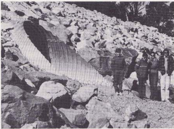
Figure 2: Photograph of the entrance to Tunnel 3. Note the size of the tunnel and the expanse of cleared ground at the tunnel entrance.
