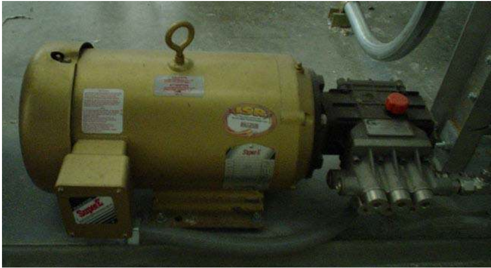
Figure 8-7 Feed Water Pump and Electric Motor
