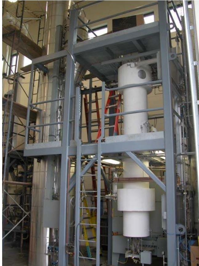
Figure 8-3 Photograph of the MASLWR Test Facility at OSU
