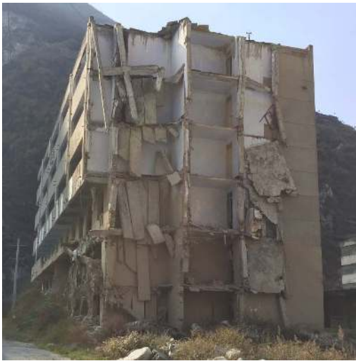
Figure 6: Flow-type slide damage in Qipan gully to a residential building
