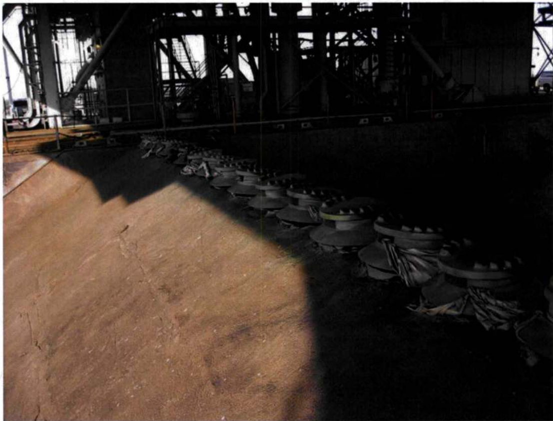
Figure 2: MFD Water Nozzles.
