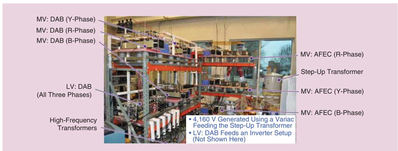
FIG 1 An experimental setup of the TIPS system at the North Carolina State University (NCSU) FREEDM System Center.
