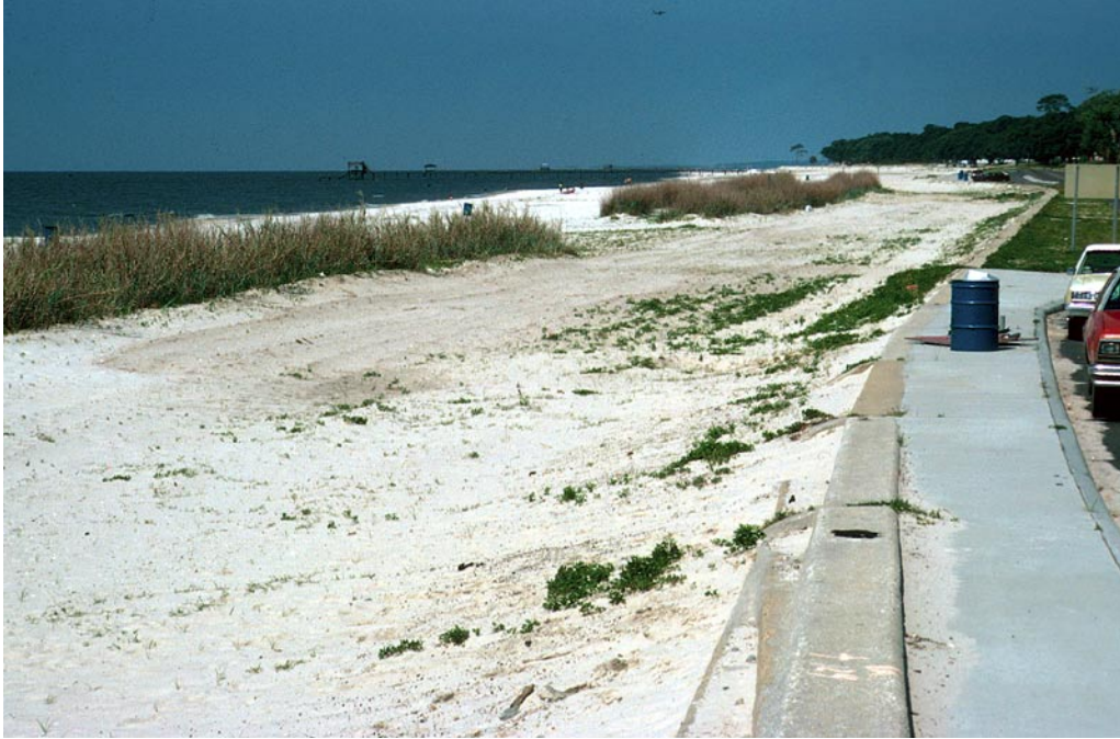
Figure 19. The seawall along U.S. 90 at Biloxi, Mississippi extends for nearly 27 miles. This reinforced concrete structure provides protection from minor storms and high water but it was unable to prevent massive destruction and death caused by Hurricane Camille in 1969.
