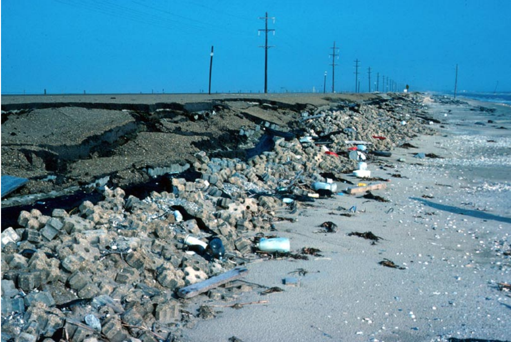
Figure 24. Storm waves in the Gulf of Mexico destroyed the interlocking block revetment constructed to protect Louisiana State Highway 82 near Peveto Beach (Fig. 3). The revetment structure was replaced with 85 segmented breakwaters between Constance Beach and Holly Beach (Fig. 3).
