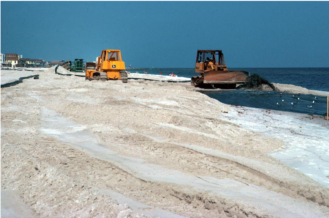
Figure 18. A beach nourishment project near Gulf Shores, Alabama. Accelerated erosion in front of the beach houses was attributed to construction of an artificial channel and jetties.
