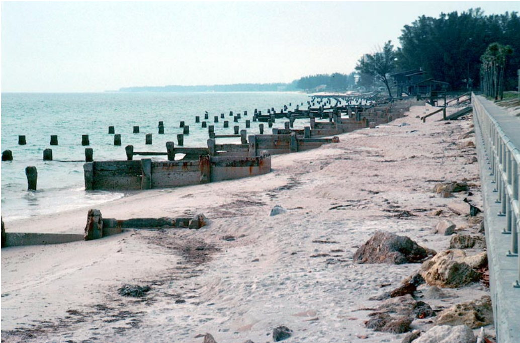
Figure 21. Multiple structures including a seawall, riprap, and failed groin field have been unable to stop erosion at Longboat Key, Florida. Later these structures were removed and the beach was nourished.
