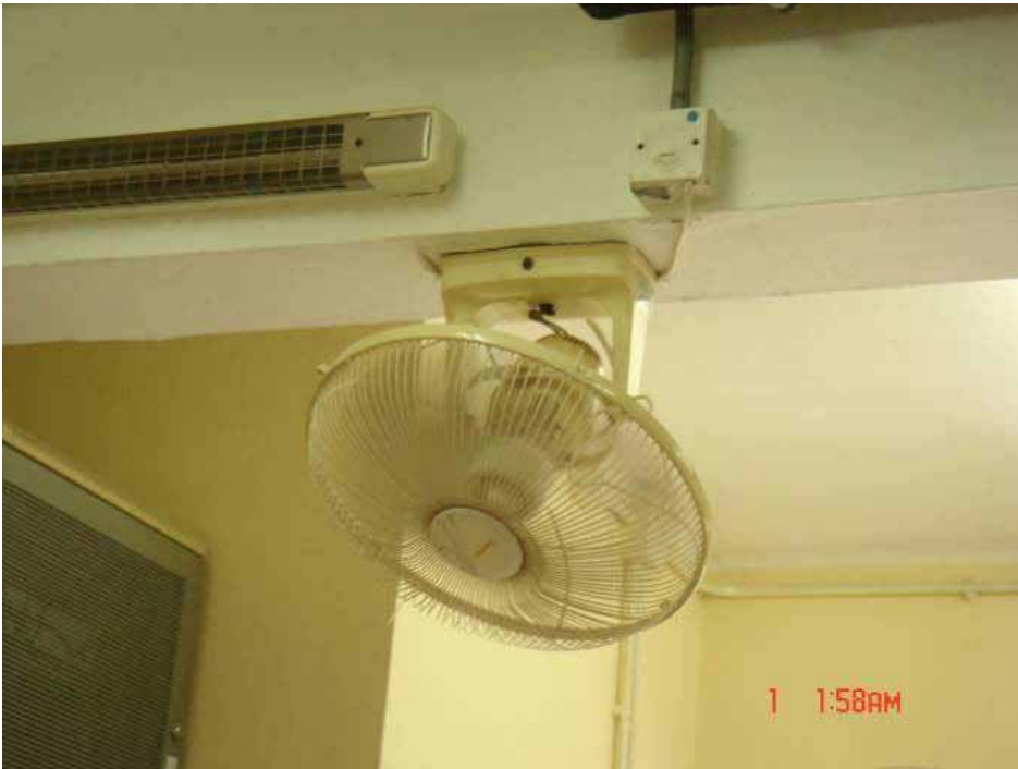
Figure G.2 A ceiling fan for summer cooling and a radiator for winter heating
