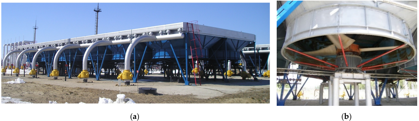
Figure 1. Gas cooling plant (a) and VASO-16-14-24 electric motor with a fan on shaft (b).
