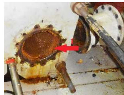
Figure 11. Seat of the flange of the freshwater cooler of the LT contour for cooling auxiliary mechanisms on a container ship MERWE TRADER (position 1 – side wall)
