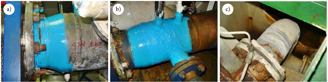
Figure 9. Repair pipe SW (sea water) line for cooling LT (low temperature) contour by comp. materials as Wet Wrap technology of container ship MERWE TRADER (in this case, fiberglass impregnated with compositions based on modified epoxy resins was used)
