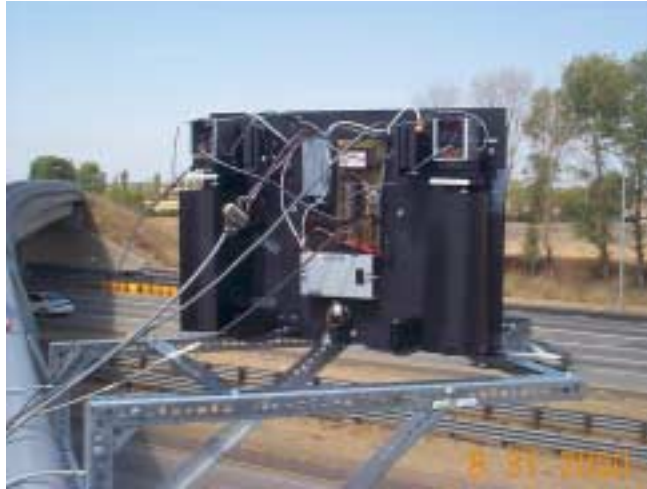
Figure 4.1: Detection System Mounted Above the Highway
