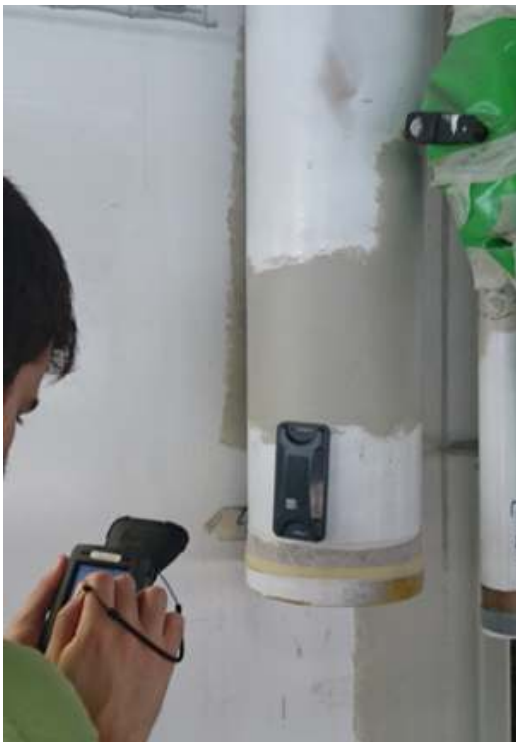
FIGURE 10: Testing of a passive RFID tag attached to one of the main pipes of the ship block.
