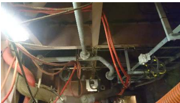
FIGURE 4: Mounted pipes on the ship ceiling.
