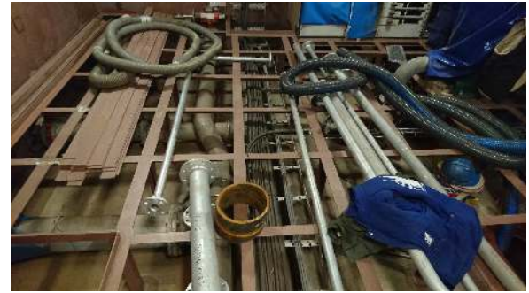
FIGURE 5: Pipes under metal floor.
