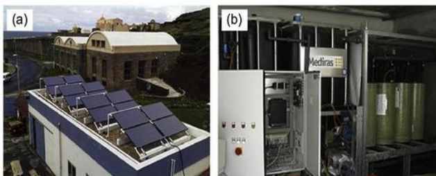
Figure 7. MEDIRAS project MD pilot plant installed in Pantelleria [26]
