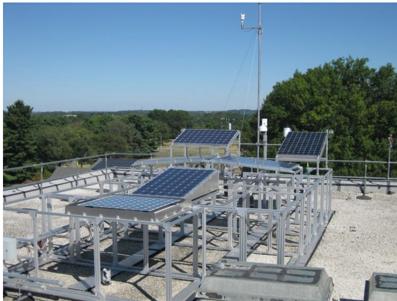
Figure 3-8 The reference modules installed at the weather station
