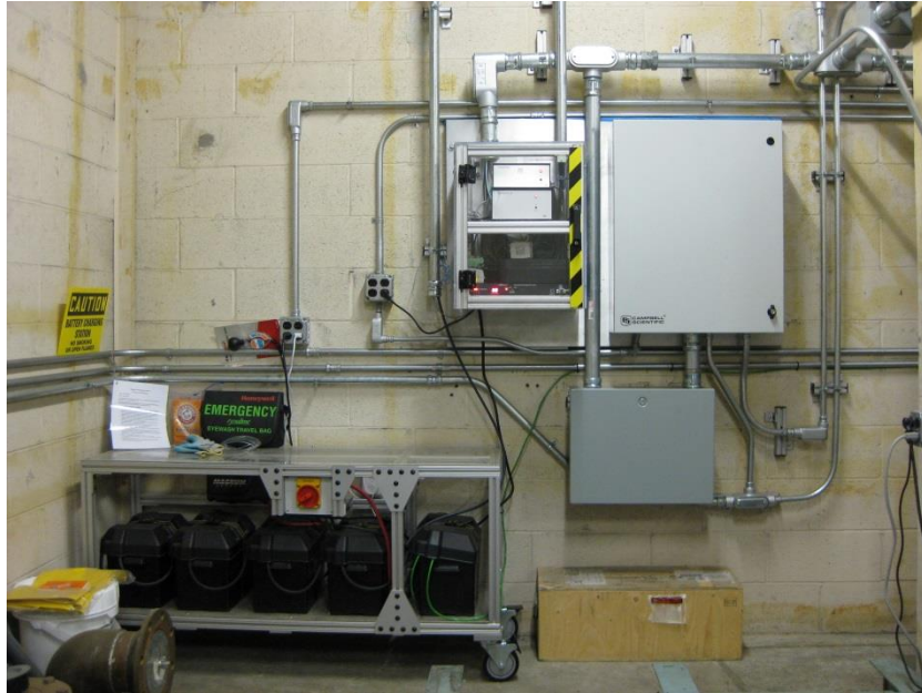
Figure 4-2 Location of the data acquisition enclosures and central UPS
