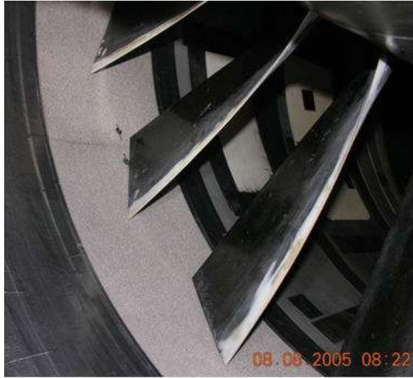
(a) Acoustic treatment mounted over the fan
