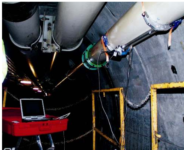
Figure 16 : Tofd equipment used to monitor the eventual corrosion on Transmanche Tunnel + cooling pipes
