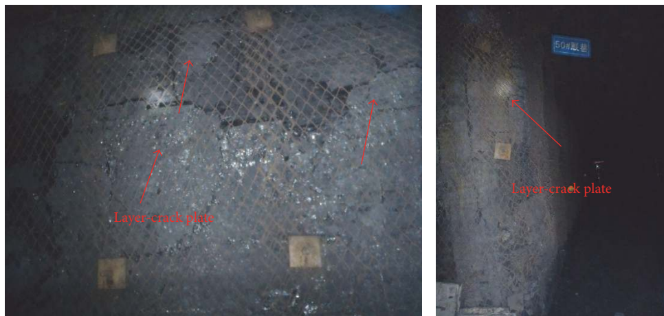
FIGURE 2: Layer-crack plate structure of the roadway coal wall.
