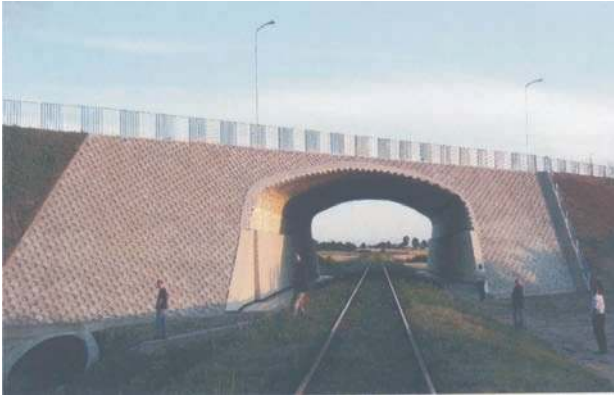
Fig. 2. Side view on the road viaduct made from steel corrugated plates situated over railway line in Prudnik, Poland
