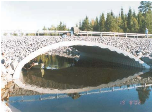
Fig. 5. Side view on the soil-steel bridge made from corrugated plates (in Sweden) (Manko, Beben 2008)
