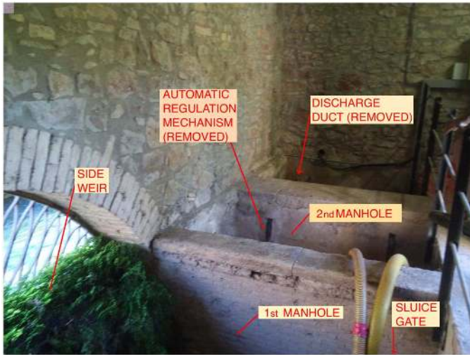
Fig. 5. Inside the hydrometric module building. (Image by authors.)
