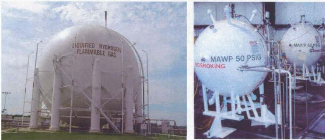
Figure 1: Liquid Hydrogen Tank in LC-39A and Demonstration Tanks at Kennedy Space Center
