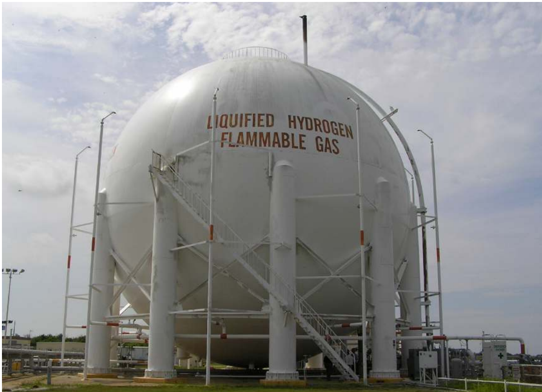
Figure 1. Liquid hydrogen tank in LC-39A at Kennedy Space Center.
