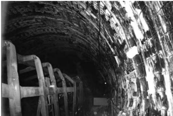
Figure 1. Fire damage in Channel tunnel
