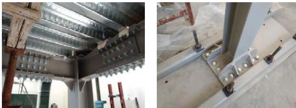
Figure 2: Detailing at the beam-column joints (left) and column base (right) of the test frame.
