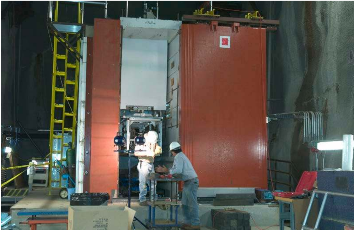
Figure 23. NuMI Workcell for hot handling operations and failed component replacement. Image shows NuMI target module in the workcell for a hot handling procedure dry run during NuMI construction
