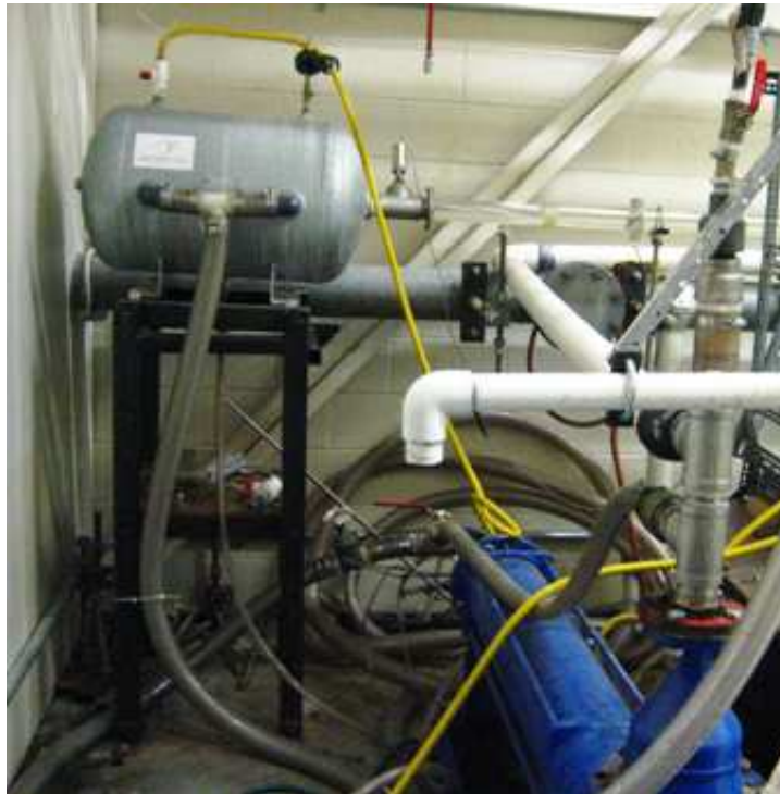
Figure A.1: Image of the reservoir tank R1
