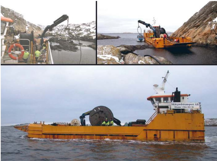
Figure 4.2: Some pictures from the installation of the sea cable which today connects the substation to the measuring station on island Härmanö.
