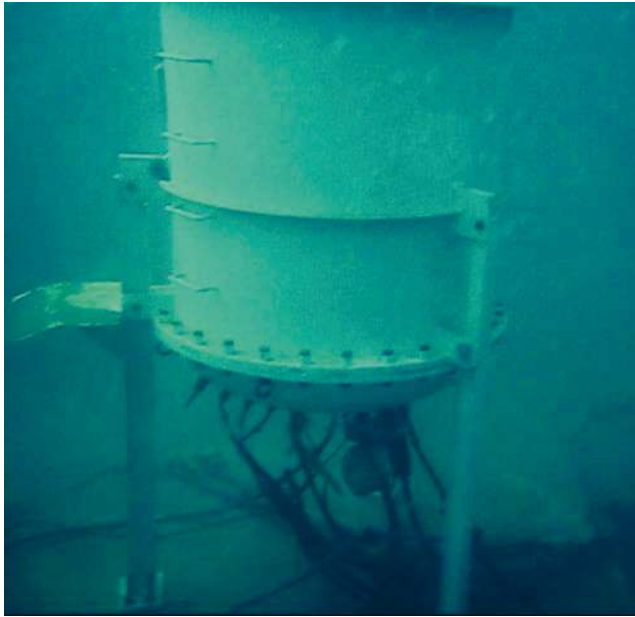
Figure 4.6: The underwater collector substation standing on the seabed.
