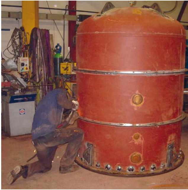
Figure 7.2: Construction: external reinforcements being welded to the hull of the new substation.
