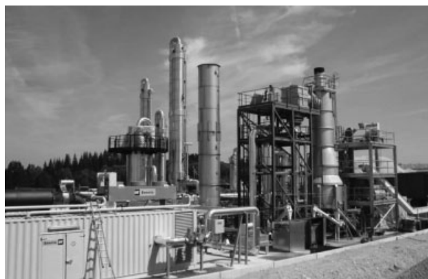
Figure 16. 1.1 MW e PRMe gasifier with OLGA in France.
