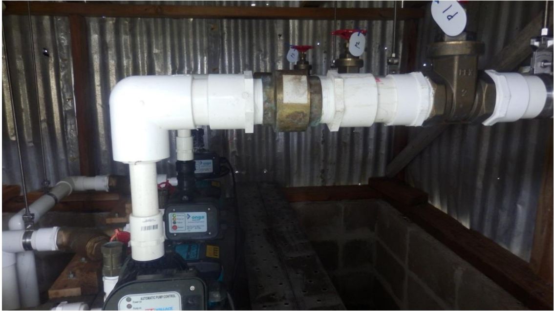
Figure 5.6: Underground water system at MSS – electric pump that pumps water from well up to overhead tanks.
