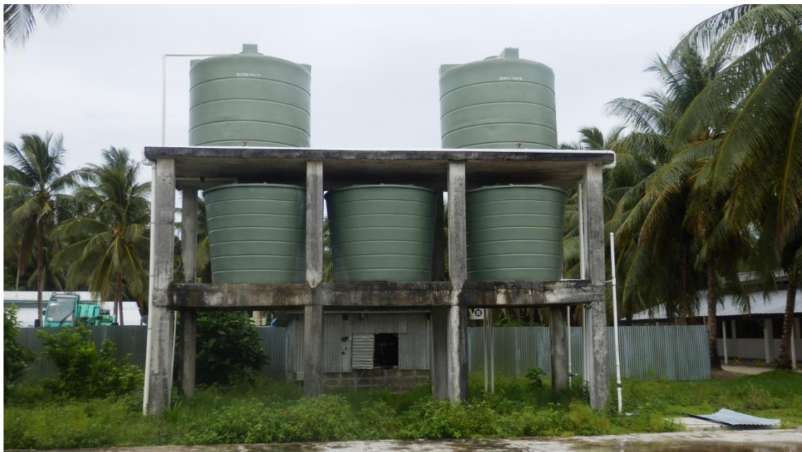
Figure 5.7: Underground water is pumped into the overhead tanks, which distribute water to students' bathrooms and toilets.
