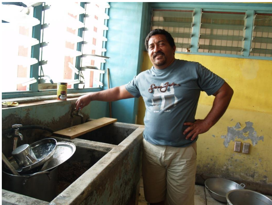
Figure 5.9: The deteriorated MSS kitchen - it needs total renovation and upgrading – 2011.
