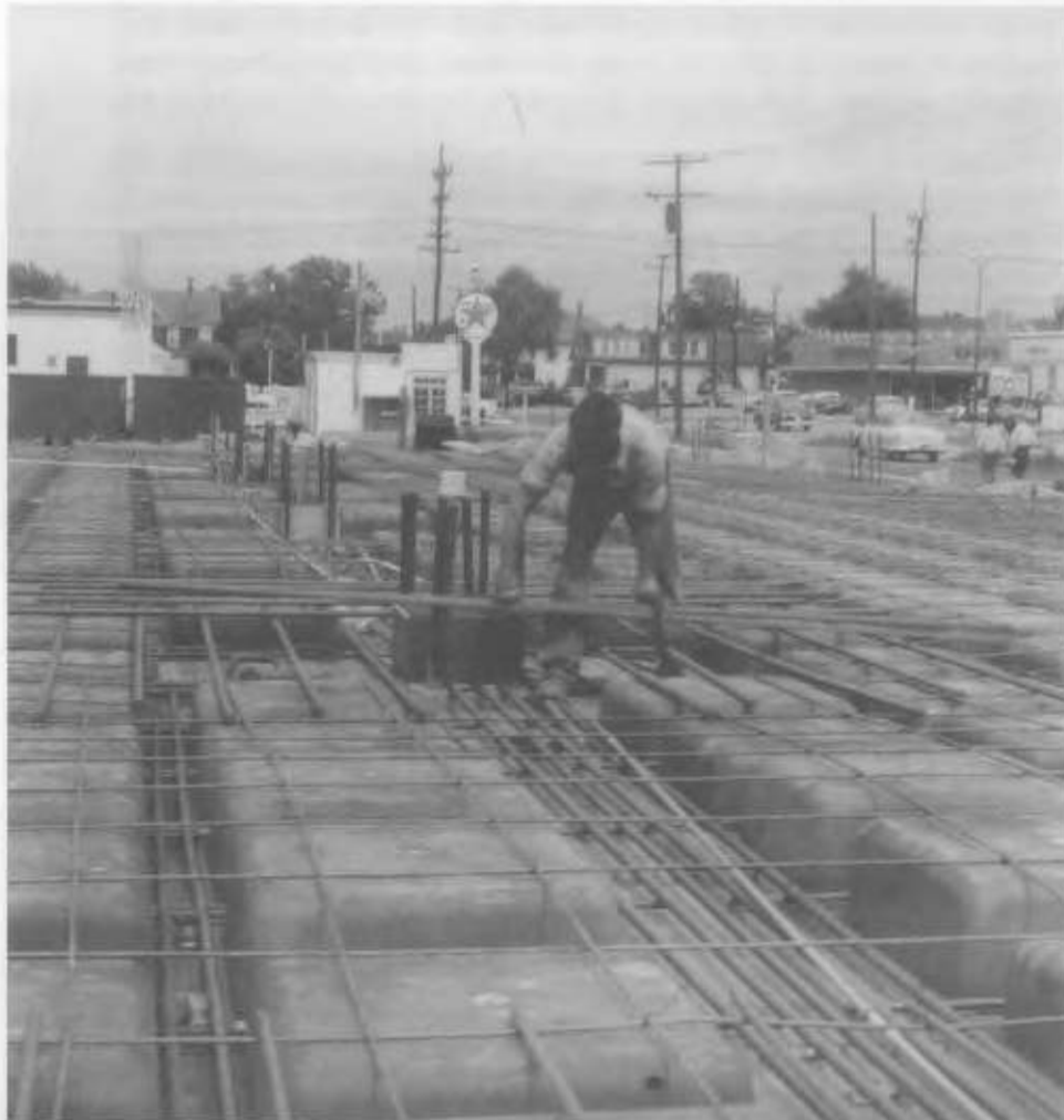
Construction under way on new Library Building located on north side of 48th Street, 1958.
