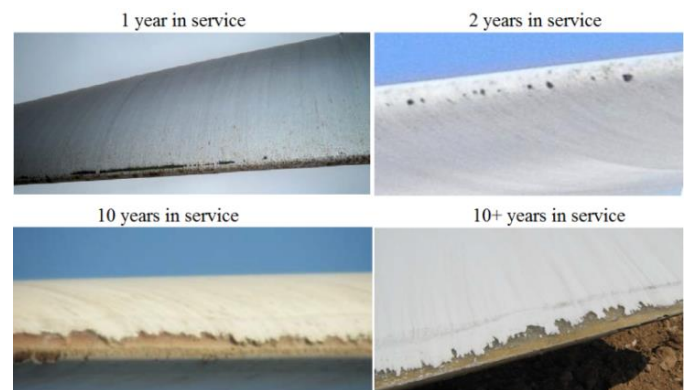
Figure 6. Examples of leading edge erosion in the field across a range of years in service. Source: [25]
