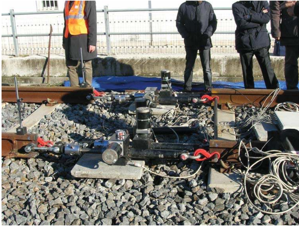
Figure 10. First longitudinal pull test: details of the actuators and their connections to the rails.
