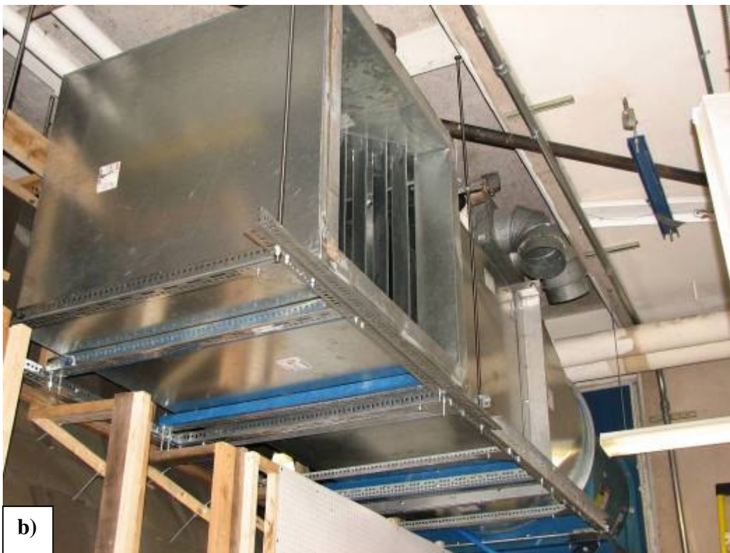
Figure A-9: Forward flight duct at different stages of the assembly process.
