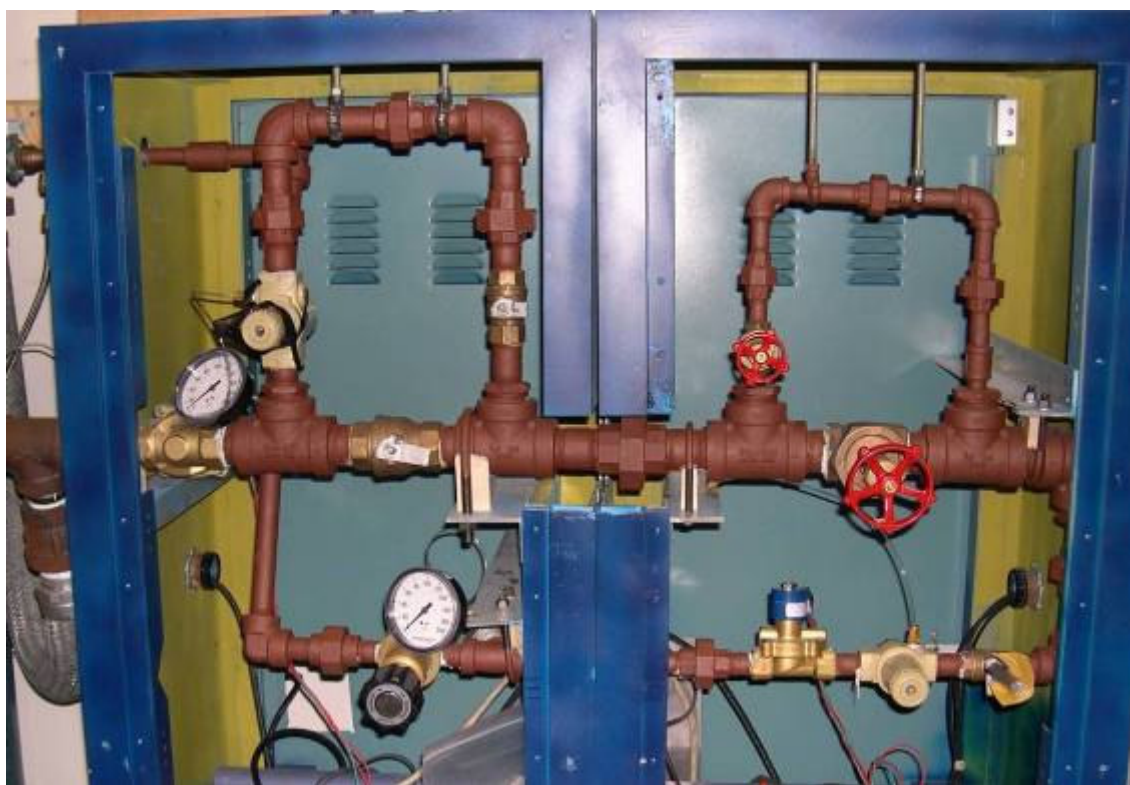
Figure A-5: Piping inside the cabinet
