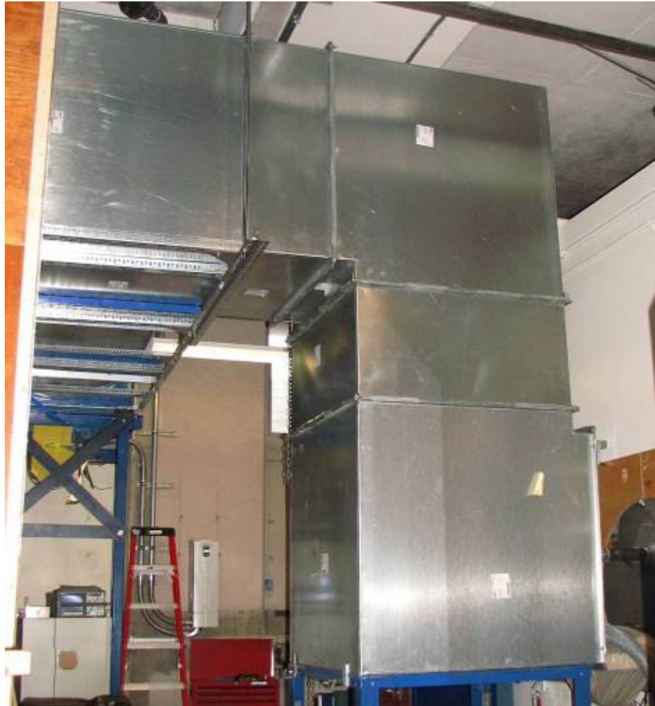
Figure A-8: a) forward flight duct as of November 2008. b) yet to be installed forward flight nozzle and inlet to the fan.
