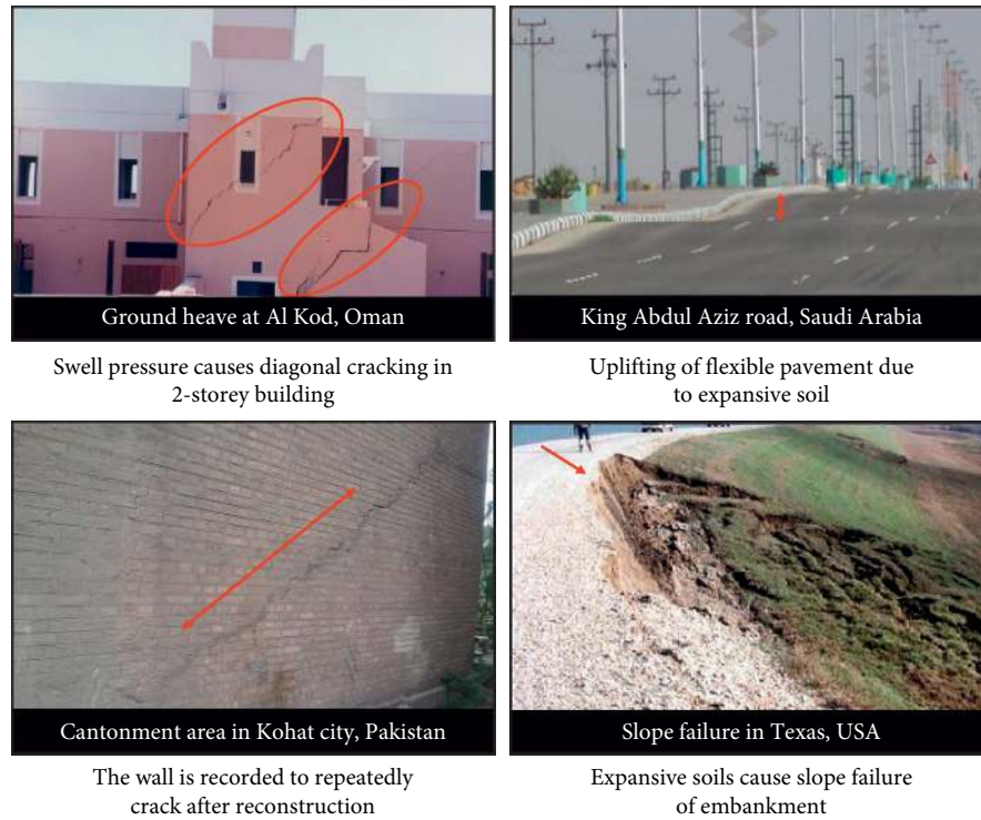
FIGURE 3: Expansive soil damage to civil engineering infrastructure across Oman, KSA, Pakistan, and USA (with some changes for comparison purpose) [62, 69–71].
