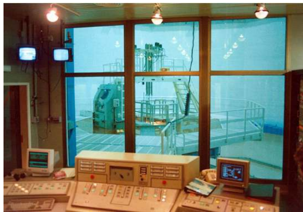
Figure 1. Control room of the Nur Research Reactor ( www.invap.com.ar ).
