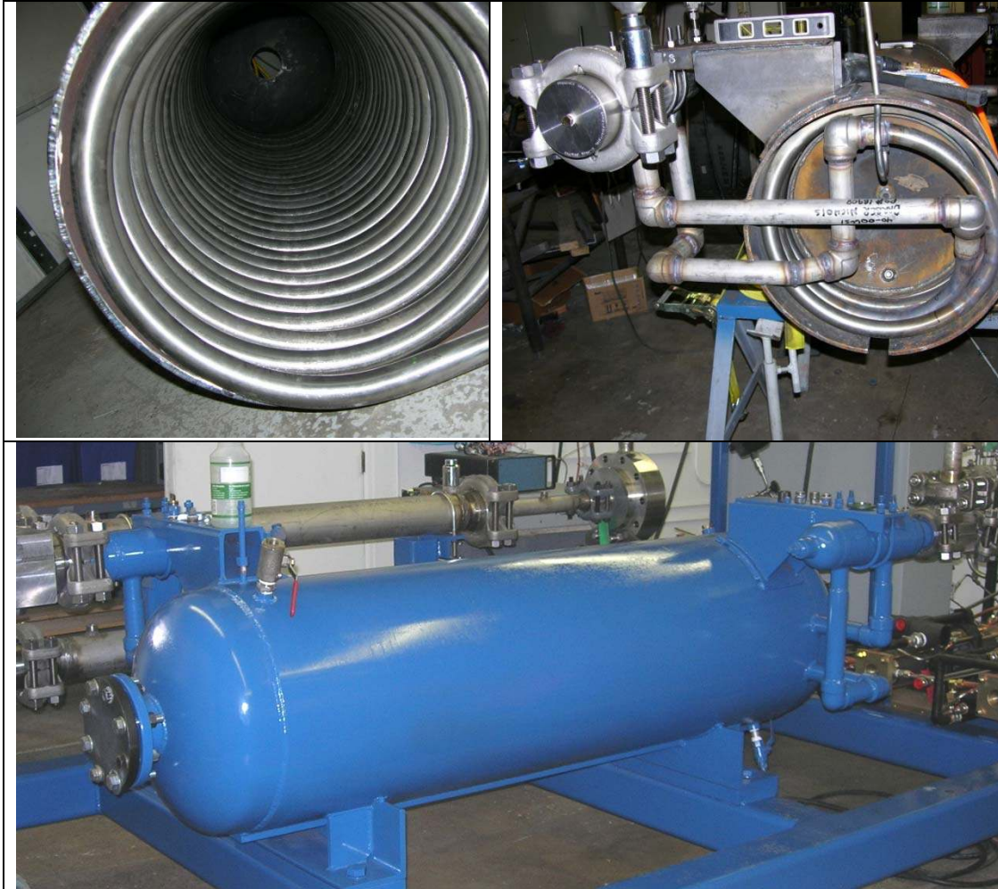
Figure 3-9: Photos of the small BNI fabricated gas chiller. The top photos show the CO 2 tubes coiled inside the water jacket and end fittings. The bottom figure shows the completed gas chiller installed on the compression loop skid.
