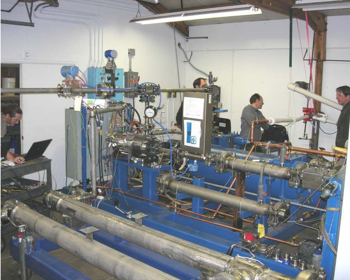
Figure 2-8: Photo of the heated, but un-recuperated, Brayton Loop. The foreground shows the heaters, the back ground shows the modified S-CO 2 test loop with the turbomachine configured as a turbo-alternator-compressor.
