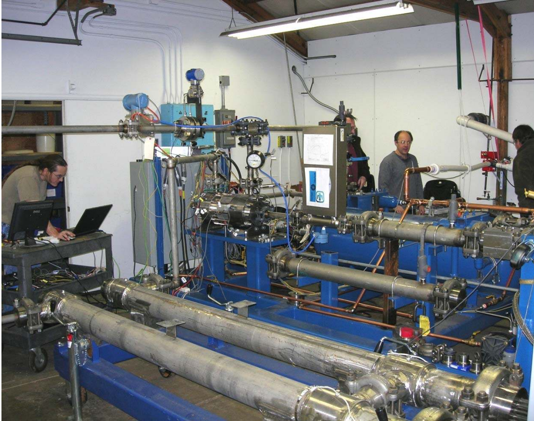
Figure 5-33: Photograph of the heated but un-recuperated S-CO 2 Brayton loop. The foreground shows the two 130 kW (each) heaters. The turbo-machinery test skid is shown in the background. The display for the data acquisition and control system is shown on the cart.
