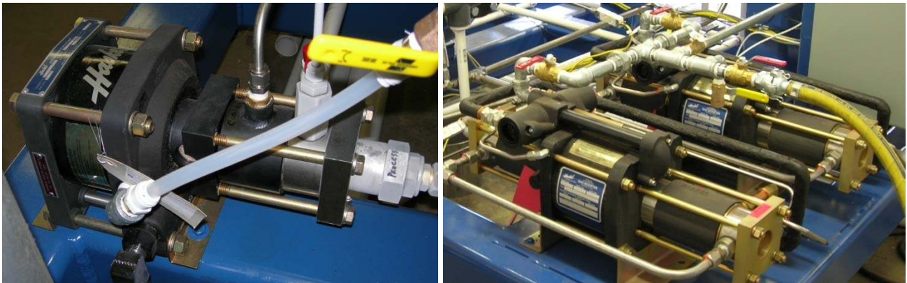
Figure 3-5: Pictures of the Haskel pumps on the SCO 2 loop.
