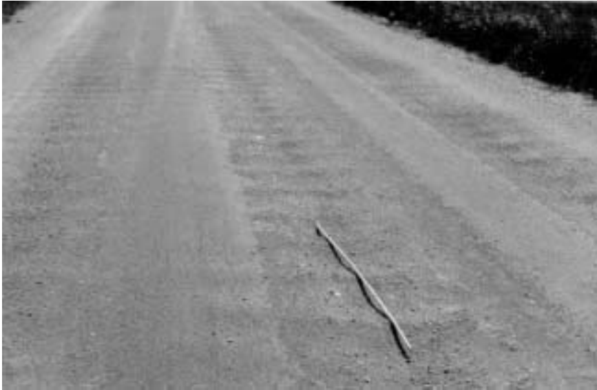
Figure 4.13 Corrugation (Chong and Wrong, 1989).
