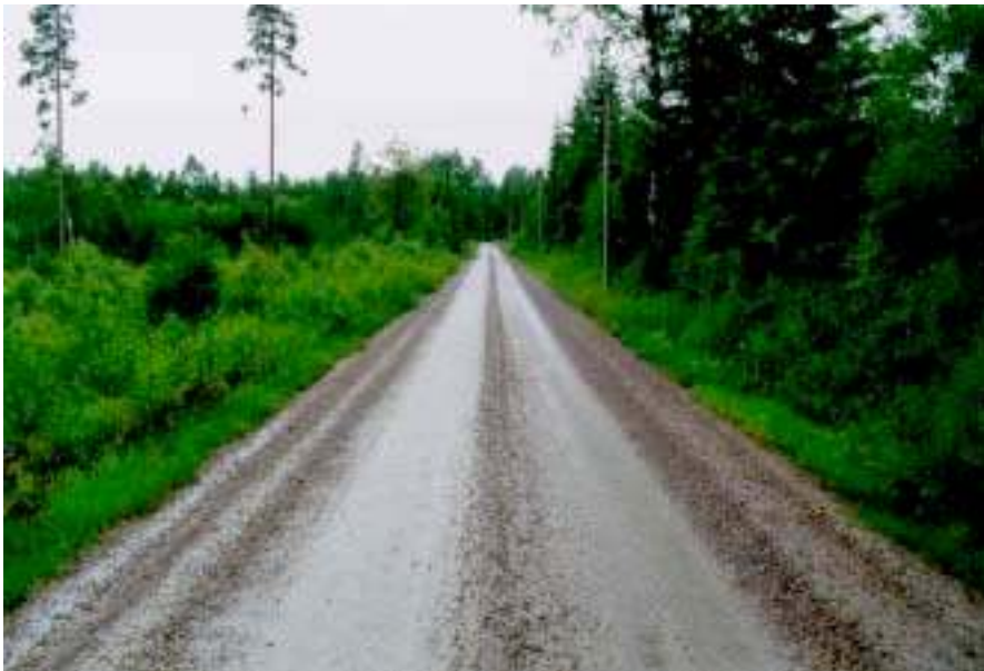
Figure 4.23 Loose aggregate on the road.
