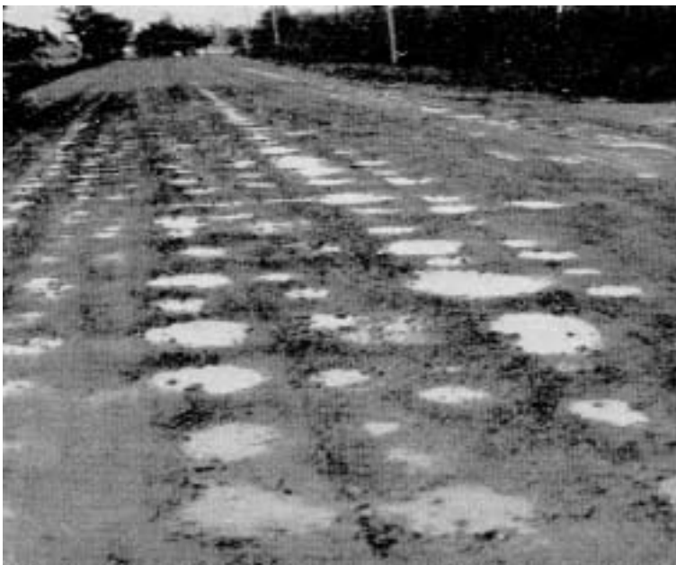
Figure 4.17 Transitional form between regular and irregular potholes (Beskow, 1932).
