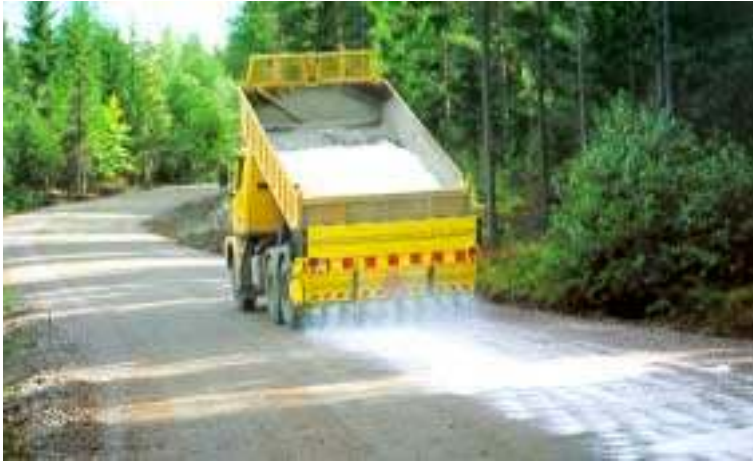
Figure 7.2 Dust control treatment with a sand spreader (Maintenance of gravel and earth roads, 1994).
