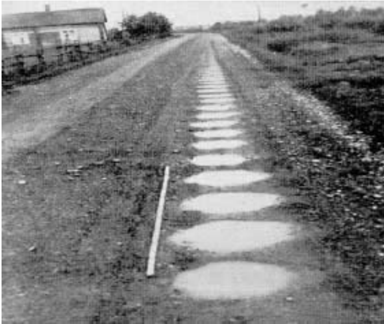
Figure 4.16 Potholes in a regular pattern (Beskow, 1932).
