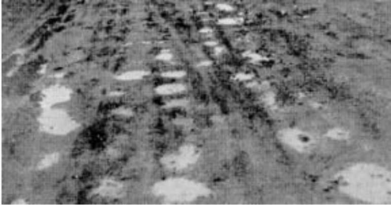
Figure 4.18 Potholes in an irregular pattern.
