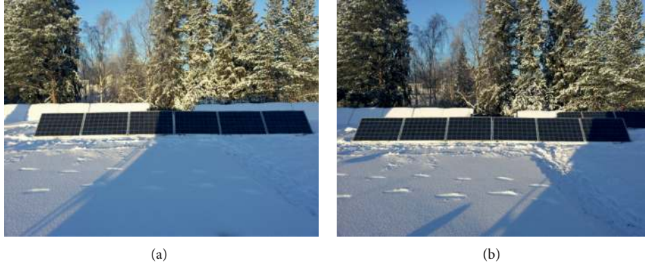
FIGURE 13: Figures of the operational conditions of String 4 under partial shading conditions caused by a building structure during the electrical measurements on December 4th, 2012: (a) conditions of measurement 1 with 2 nonshaded PV modules and 4 fully or partially shaded PV modules, (b) conditions of measurement 4 with 5 nonshaded PV modules and 1 partially-shaded PV module.
