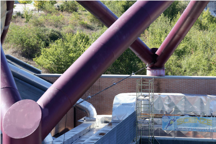
Fig. 6.25 Installation of the prototype of monitoring system on one of the cables of a sample steel arch
