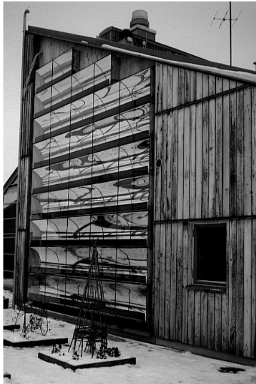
Figure 27: Facade-integrated solar thermal collectors with semi-parabolic over edge reflectors. Photo: B. Karlsson.
