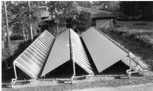
Figure 22: Solar collectors with planar reflectors of corrugated aluminium. Photo: B. Karlsson.
