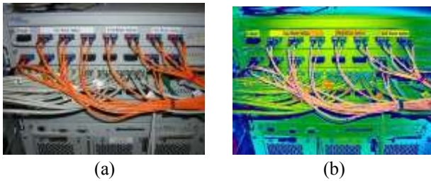
Fig. 6. Visual Inspection of optical MUX-DEMUX rear cables reveals the existence of electrical anomalies (Sample 2) a) RGB regular image, b) Thermal Image
