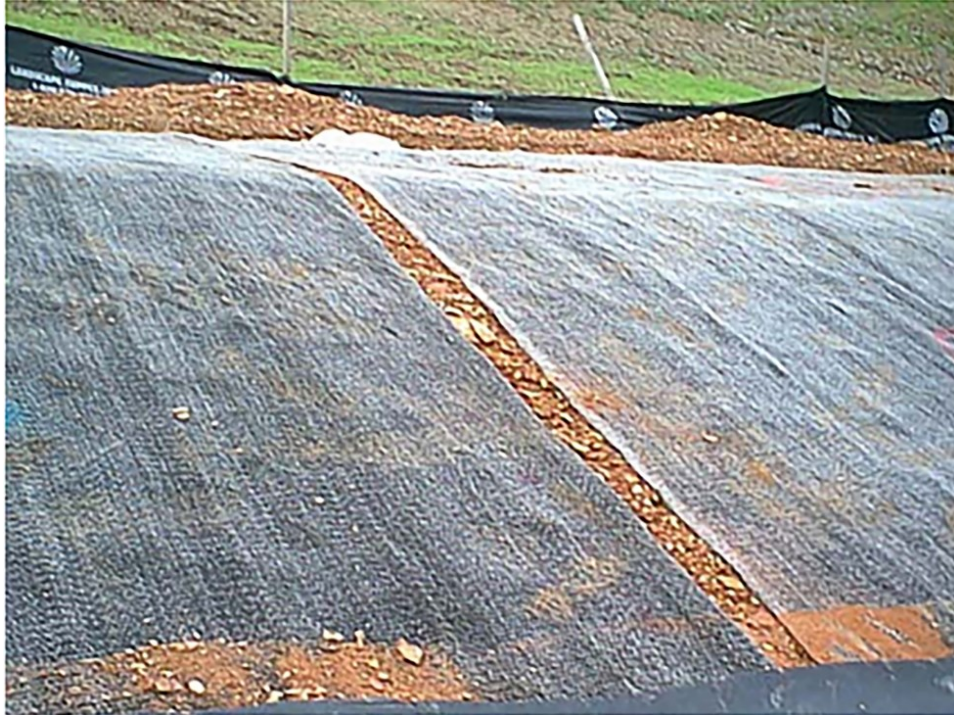
Figure 6. Photograph showing gap in GCL panels after removal of geomembrane (Thiel and Richardson, 2005)
