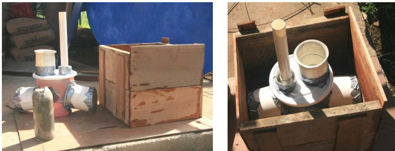
Figure 5: Wooden mold and sacrificial mold core that holds the shape of the cavity for the tensioner and bearing that sits at the bottom of the well.
