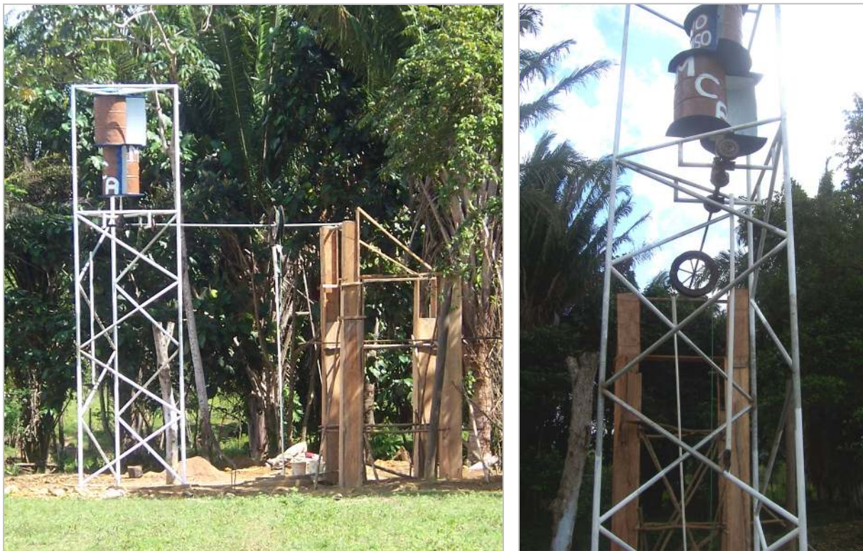
Figure 1: Two views of the wind-powered water pumping system installed on the property of the Nuevo Paraiso Enterprise in Guadalupe Carney, Honduras.
